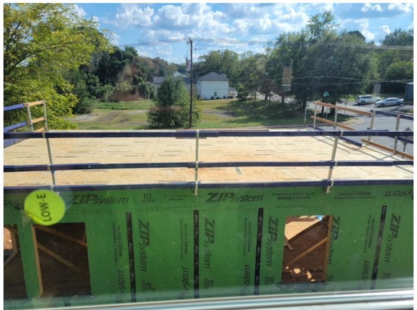
The end of the day after the 2 nd Floor Decking was installed.
