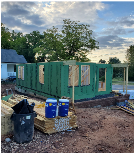
Start of the day prior to installing the floor joists for the 2 nd Floor.
